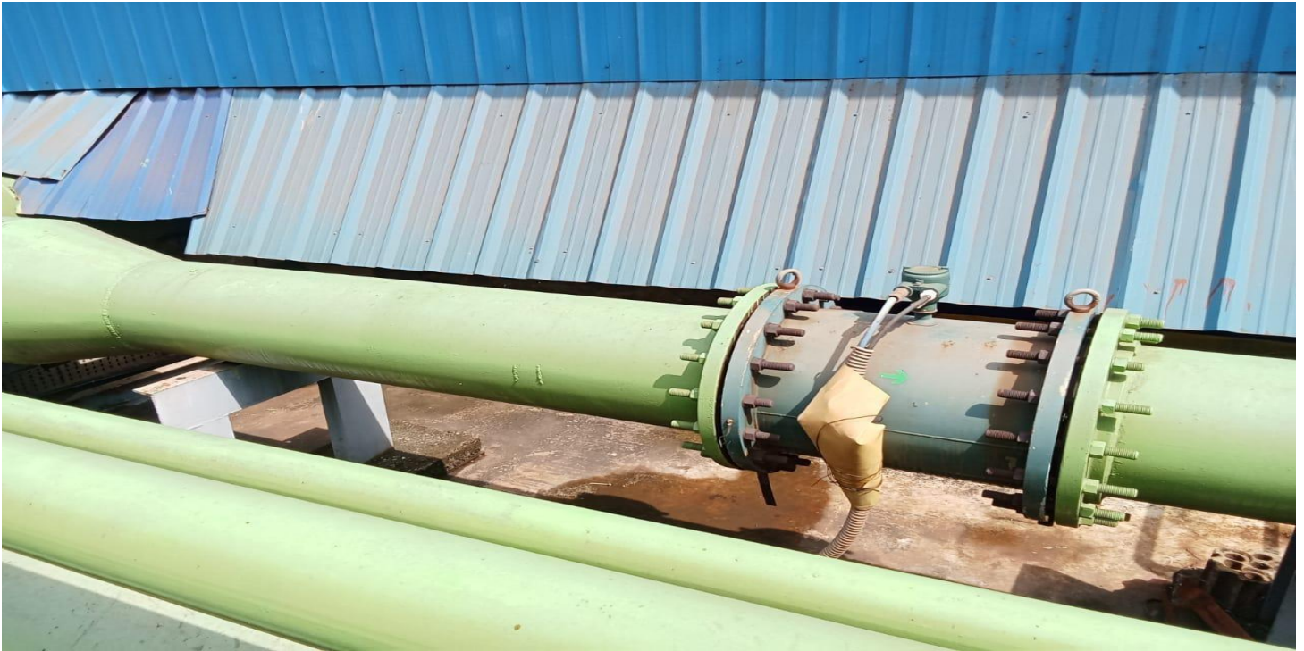
EOF Flow meter
