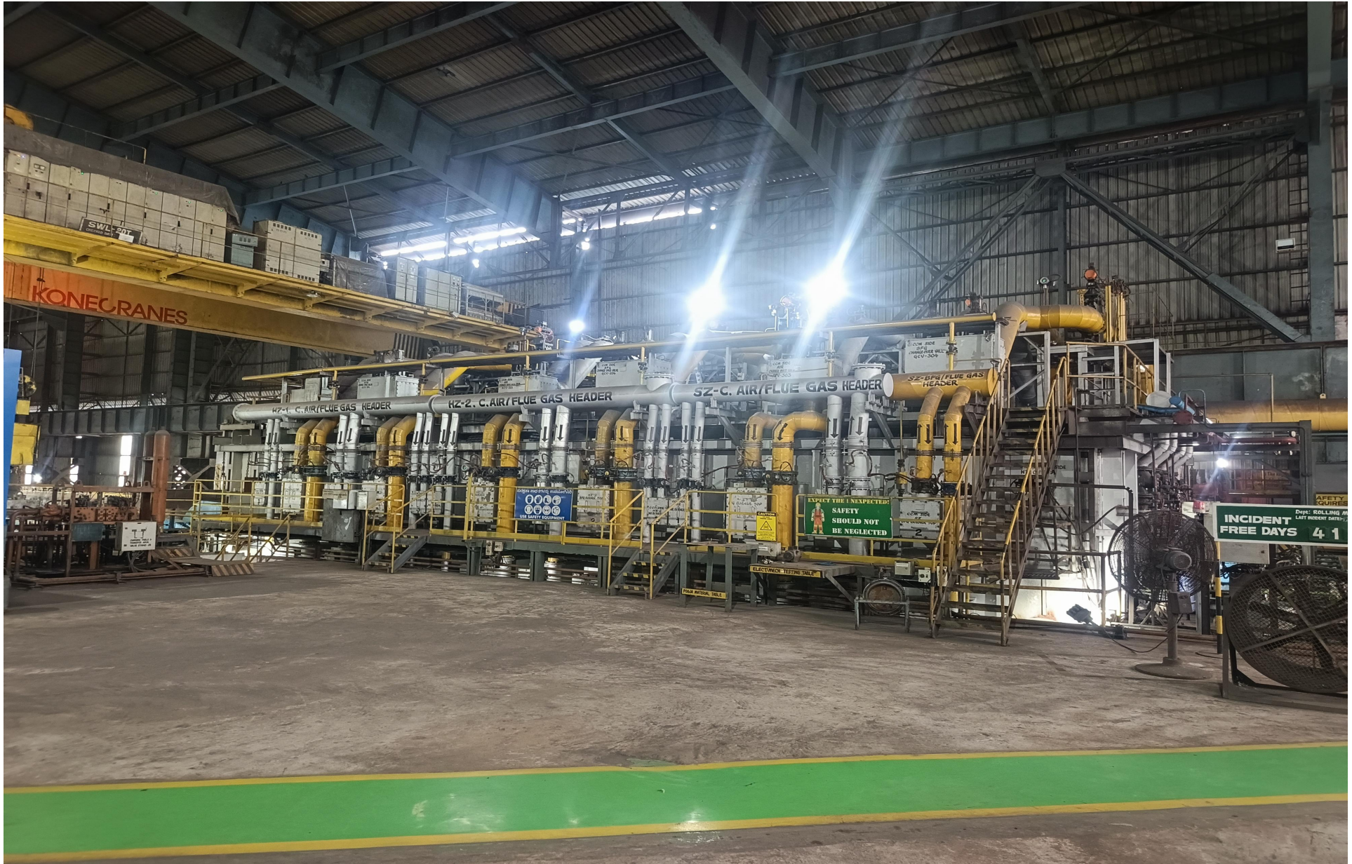
RHF Regenerative Furnace
